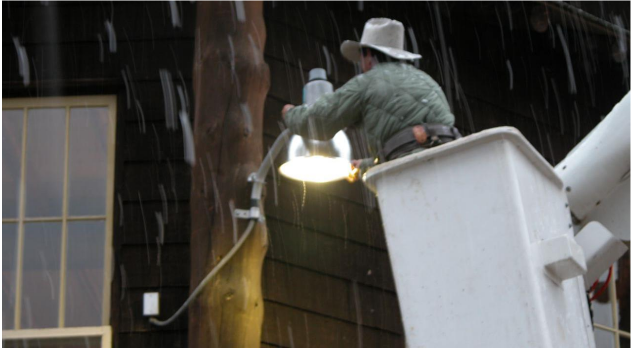
Figure 24. A full cutoff shield being installed on an existing light on the lodge at Yellowstone National Park. This previously unshielded light was visible across the lake and from the backcountry. Photograph by Travis Longcore.
