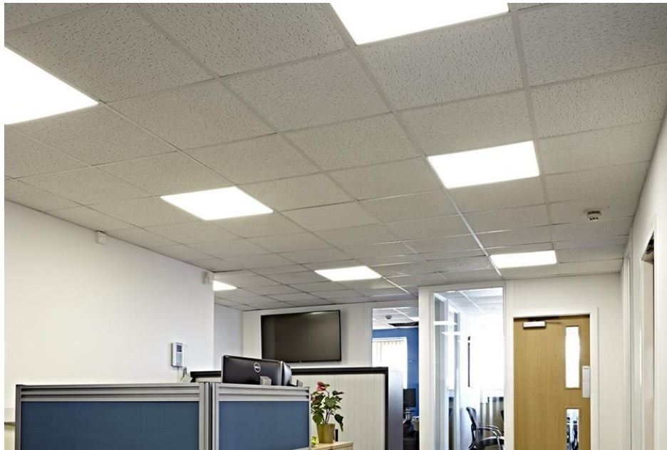
Figure 8 - LED Office Lighting
