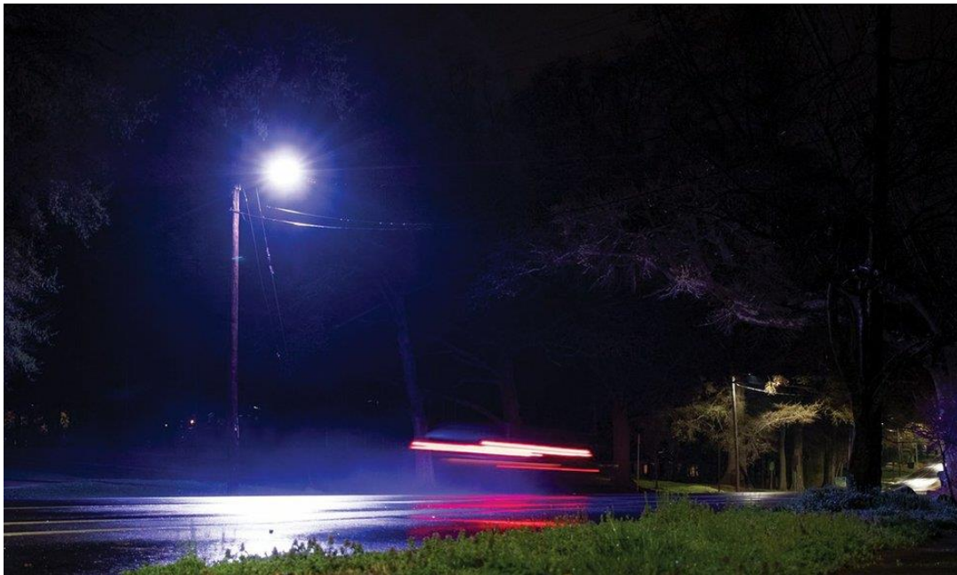
Figure 4 - Purple LED Streetlight
