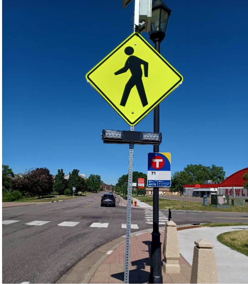
Figure 2 - RRFB at Market Place Drive
