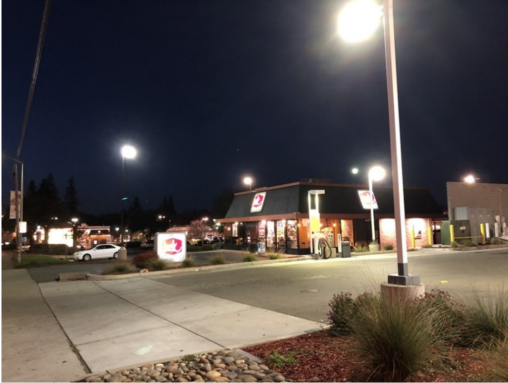
Figure 2 - LED Parking Lot Lights
