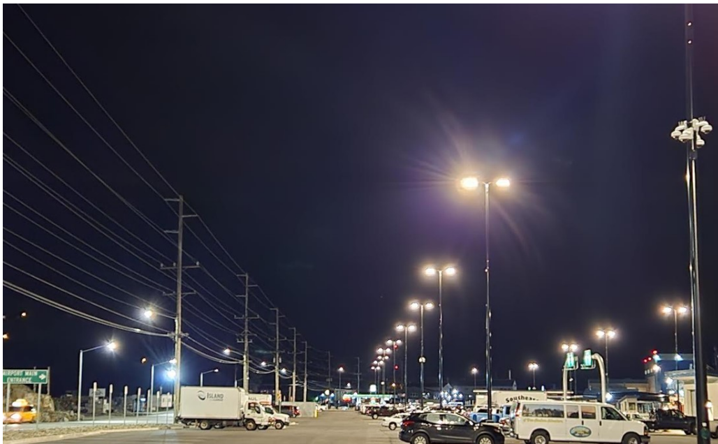
16 17 18 19 20 21 22 23 Figure 12 - LED Airport Lighting
