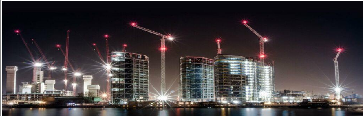
Figure 22 - LED Lights on Towers
