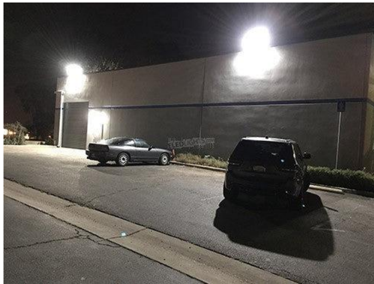
11 Figure 16 - LED Wall Pack Flood Lights
