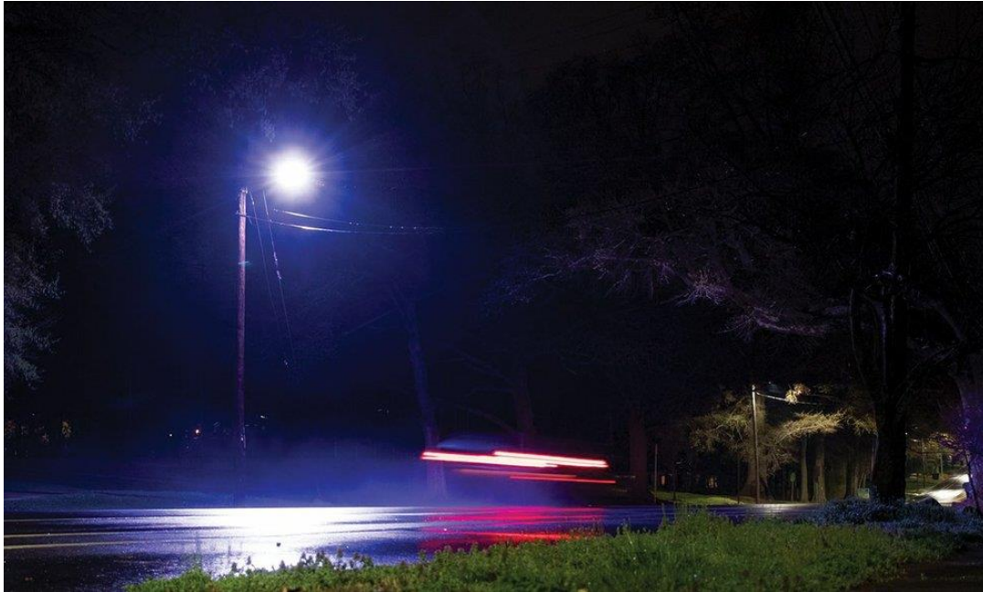
Figure 13 - Purple LED Streetlight
